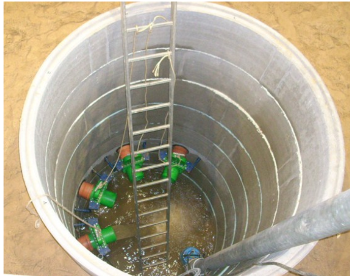
Figure 4.14: Pumping well and valves for switching on/off of the drains
