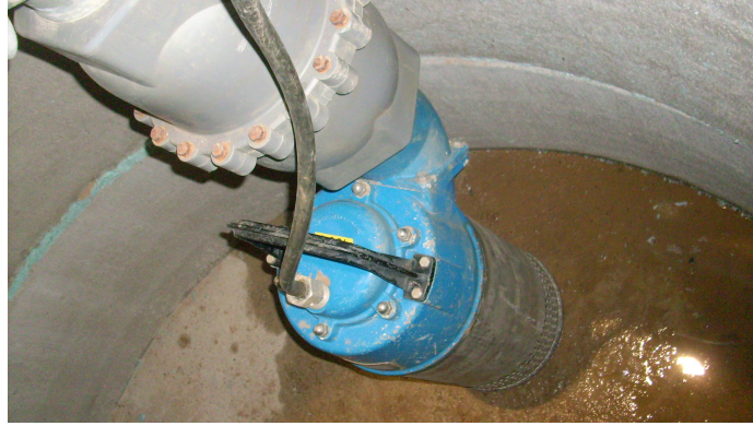
Figure 4.15: Pump placed in the well
