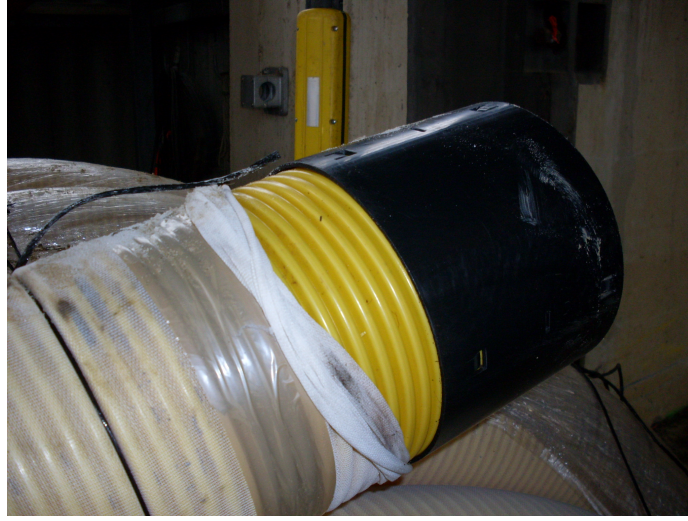
Figure 4.12: Particular of the drain pipe
