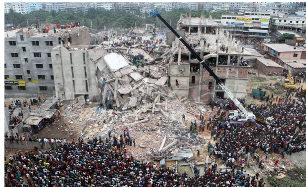
Figure 7: Rana Plaza disaster: an aerial view of the disaster zone after the building collapse
